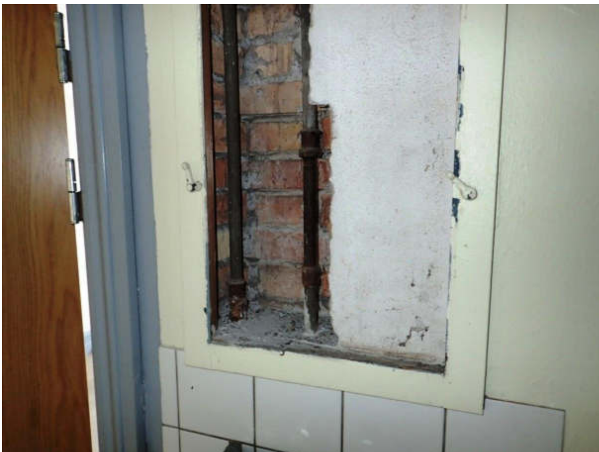
Figur 32 Lem mangler mod teknisk /installation.
